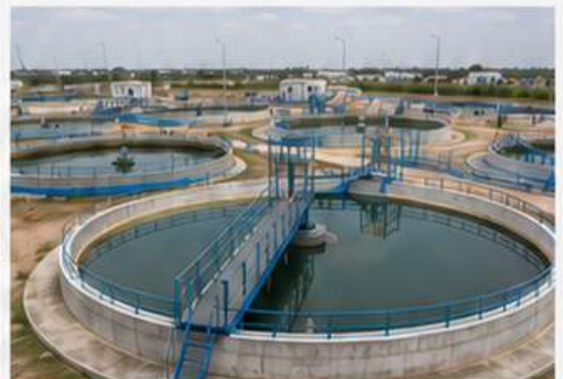
WATER SUPPLY INFRASTRUCTURE
